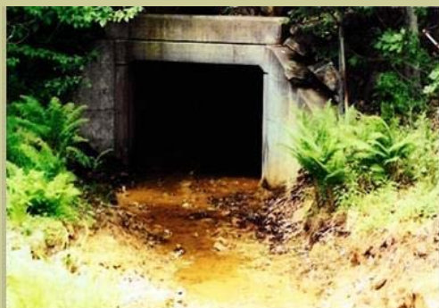
A box culvert was used to allow Jonathon Run to pass under I-80.
