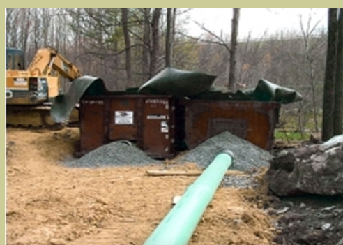
The self flushing pilot-project systems in place at Jonathon Run.
